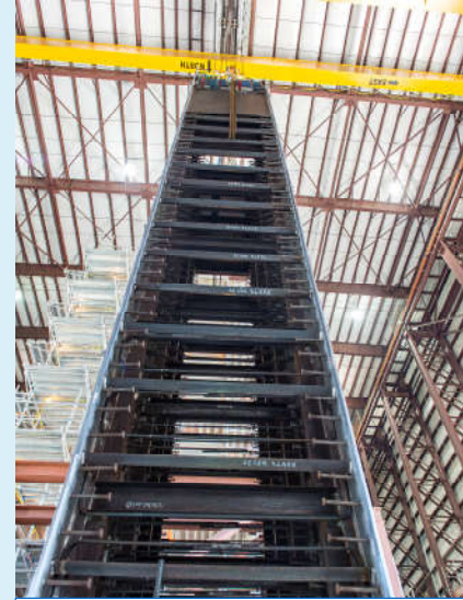
Sub-module inside the Module Assembly Building May 2015 © Georgia Power Company
