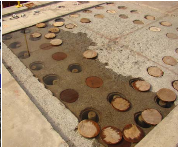
20 rods seen entirely submerged in water (Picture taken 1/12/2011)
