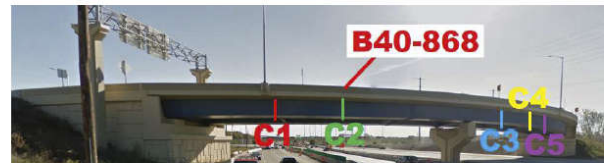
Figure 5-2 B40-868 Crack Locations
