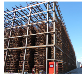
7.3 High Density Rack Storage
