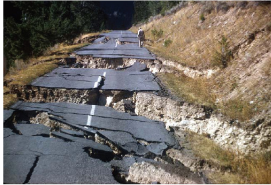
Fig. 1-9. Lateral spreading damage to highway pavement near Yellowstone Park, 1959 Hegben Lake earthquake. (Photo courtesy of U.S. Geologic Survey)
