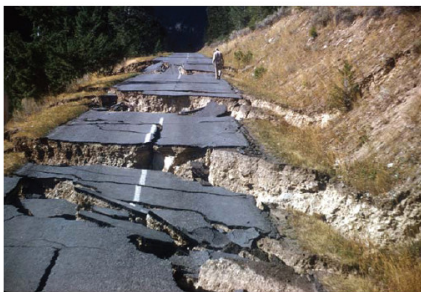
Fig. 1-9. Lateral spreading damage to highway pavement near Yellowstone Park, 1959 Hebgen Lake earthquake. (Photo courtesy of U.S. Geologic Survey)
