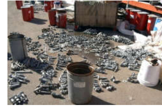
Not Properly Handled
