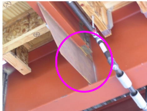
Torsional bracing provided by shallow perpendicular steel framing and stiffener - wood framing was not considered adequate
